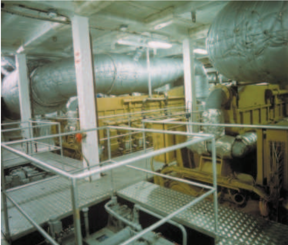
ENGINE ROOM OF THE AQUASTRADA TMV 115
